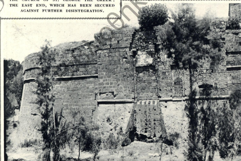
THE SOUTH-EAST FLANK OF THE GREAT RAVELIN BEFORE CONSERVATION : A SURVIVAL, DATING FROM 1544, OF THE EARLIEST ARTILLERY SYSTEM ; PERHAPS UNIQUE, SINCE SUCH EARLY FEATURES WERE GENERALLY REMOVED FROM FORTRESSES DURING LATER MODIFICATIONS.
