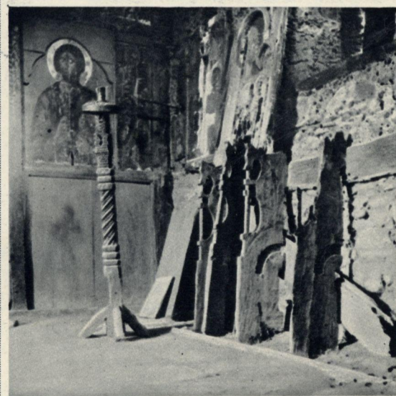
THE INTERIOR OF MOUTOULLAS CHURCH, IN DEPLORABLE DISREPAIR: MEDIÆVAL PAINTINGS WHOSE PLASTER IS FLAKING OFF OVER LARGE AREAS.
