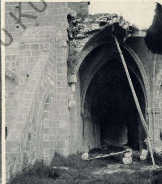
VAULTING IN ONE OF THE CLOISTER WALKS OF BELLAPAISE ABBEY TEMPORARILY SHORED UP: A THIRTEENTH-CENTURY LATIN MONASTERY.
