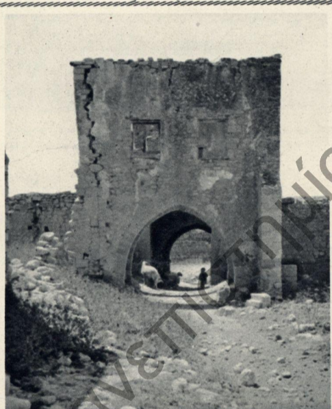
THE GATEWAY OF THE LUSIGNAN PALACE AT KOUKLIA, IN URGENT NEED OF TREATMENT: A HUGE CRACK ENDANGERING ONE SIDE.
