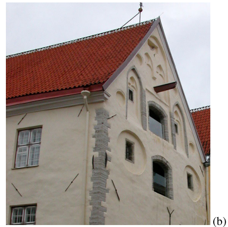
Figure 15: Tallinn: retrofitted building in old town (a), bar shaped tie rod end (b)
